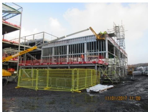
Photograph 3 Following completion of main structural steelwork the steel erector has now commenced the erection of the external mild steel starting with the sports hall
